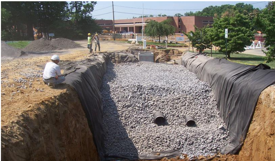
Figure 3. 13 Infiltration Trench (DCCC 2009)
